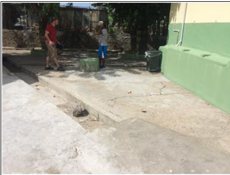
Figure 9: The primary school had a new septic tank installed within the last 2 years. It was not pumped before the tank and has not been pumped since. It appears to discharge into the open gutters.
