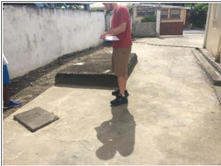
Figure 13: The wellness center has two tanks; one we were unable to locate. Effluent is believed to discharge to the soakaways on site or to the gutters.
