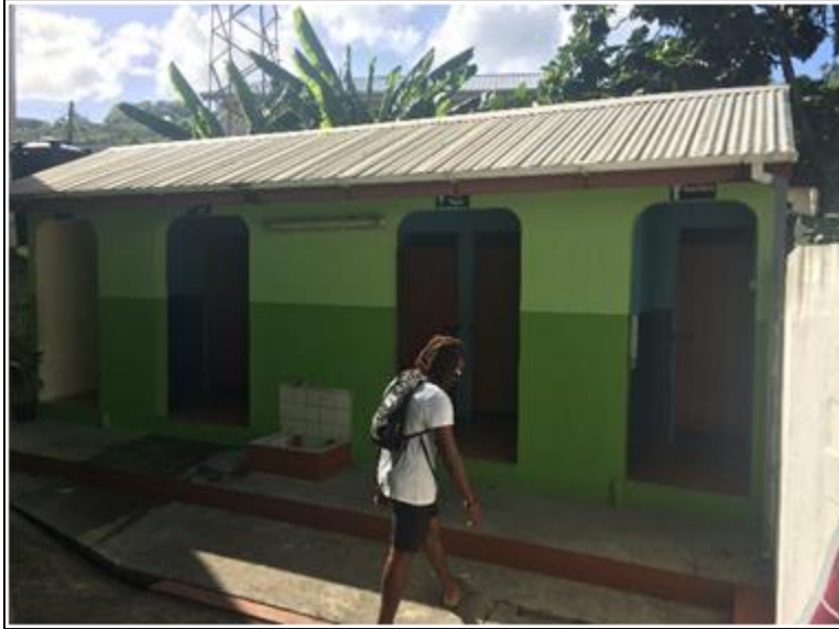
Figure 12: The secondary school is pumped every 2-3 years and has a soak-away which was not visible. Previously held 200 students, but now has 93.
